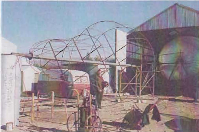
The gel coat has been applied to the apple in the shed whilst the frame work of the pear is pictured with Steve Bell in the foreground.
